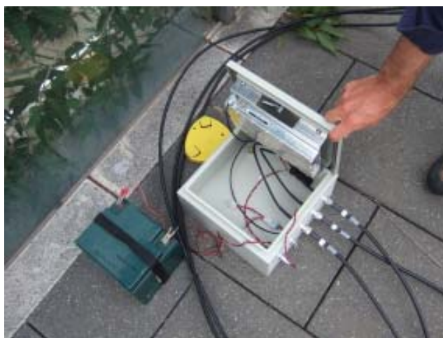
Fig. 1a. LocataLite inside box with cabling to antennas.
